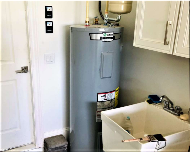
A.O Smith 50 gallon hot water heater
