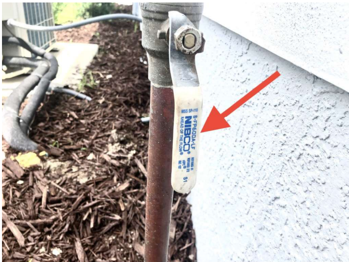
Main water shut off valve
