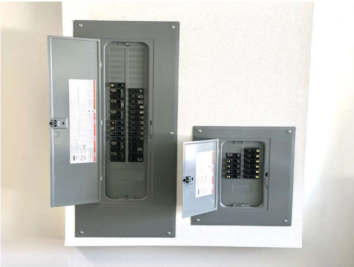
Main electrical panel (left) Sub panel (right)
