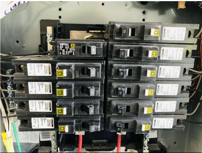
Sub service panel
