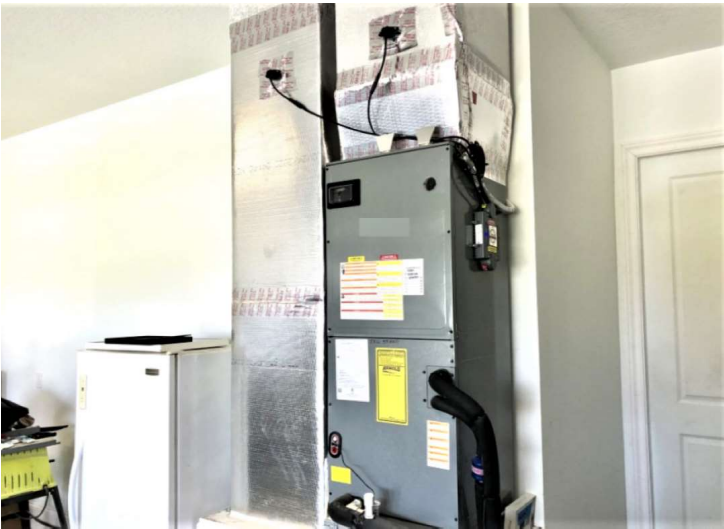
Matching air and heating unit located in the garage
