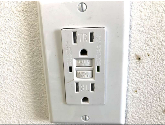
GFCI breakers located in all wet areas - Arch flash relay's located at breakers
