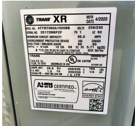
Outside air conditioning unit label - MFD 4/2020
