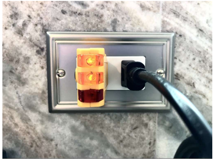
Polarity tested satisfactory at electrical outlets
