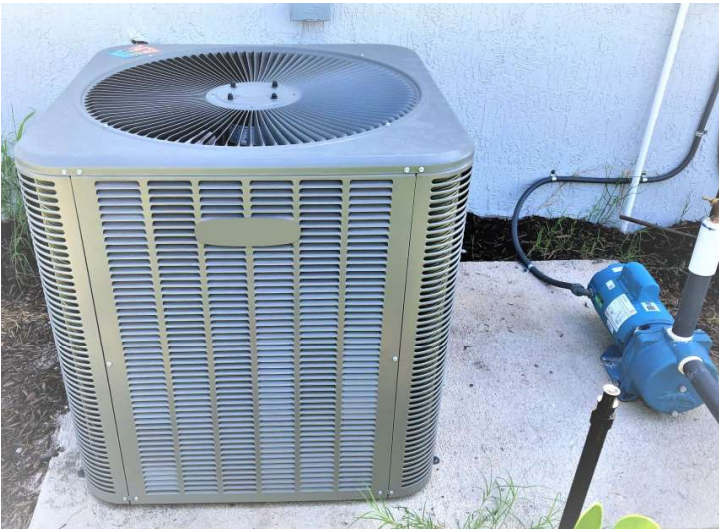
3.5 ton or 42,000 BTU outside air conditioning unit
