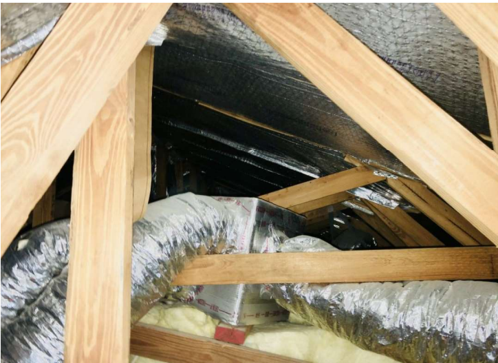
Attic insulation and air/heating ductwork adequate
