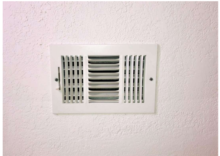
Air and heating distribution grills clean and in good working condition
