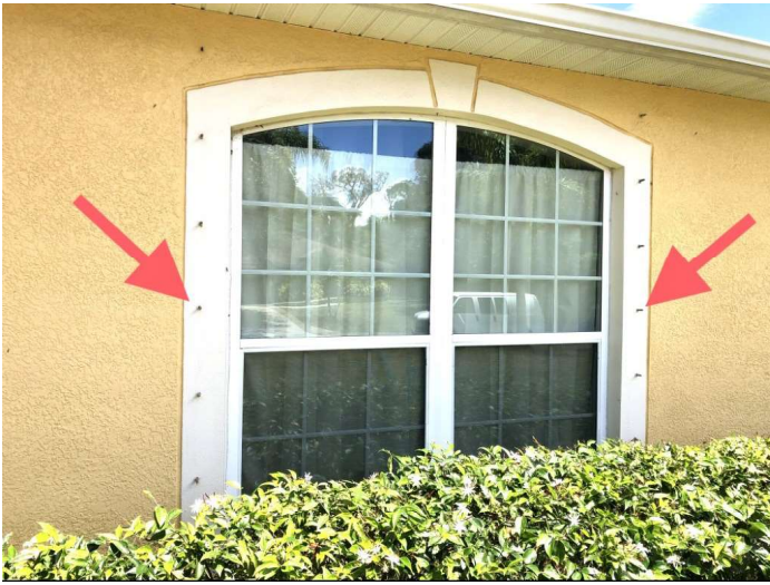
Single hung windows with shutters - hardware included (red arrow)
